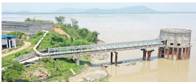
Raw Water Intake under South Central Guwahati Project
