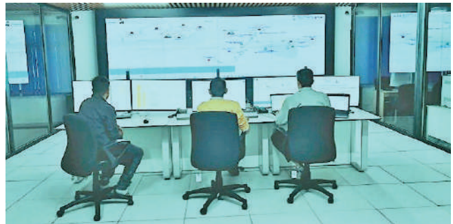
Centralized SCADA Monitoring Center installed in the GMDW&SB office
