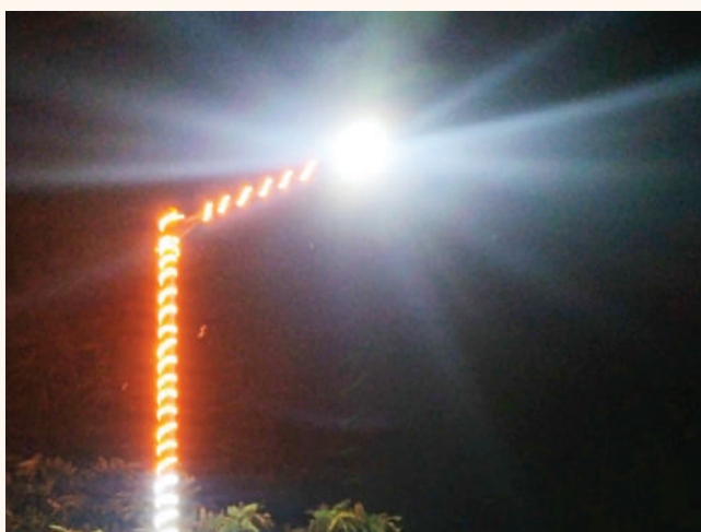
Solar Street Light
